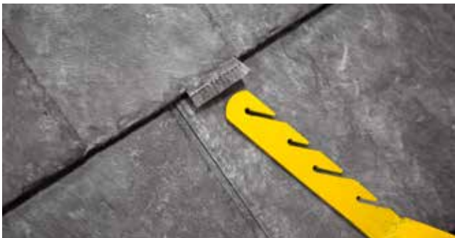
Fig. 9.3 - Roof jack removed
