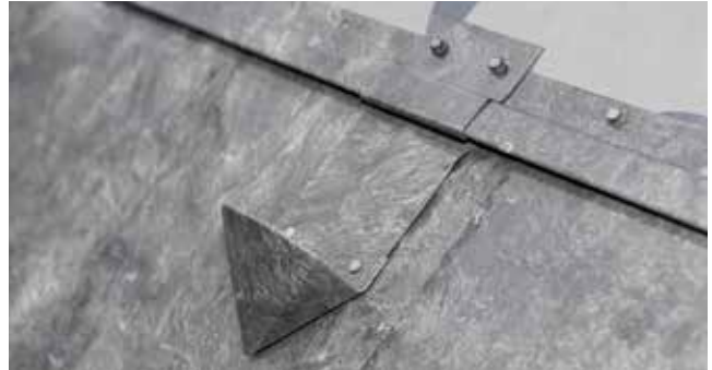
Fig. 35.1 - ProGrip diverter installed
