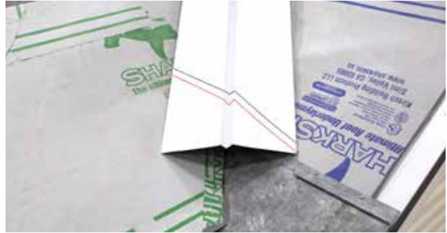
Fig. 18.1 - Valley flashing marked and ready to cut and fold Red = Cut / Black = Fold
